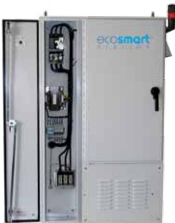
Zone 1: Service Entrance Compartment
