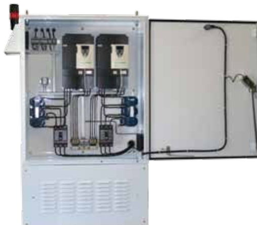
Zone 2: MCC Compartment
