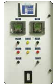
Zone 3: Inner Door of Controls Compartment
